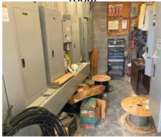
Exterior Communications Room (Female Side) Clutter
