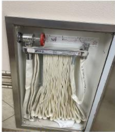
Typical hose cabinet
