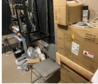
Clutter in telecommunications room
