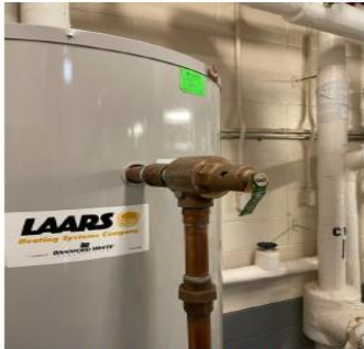
Relief valve missing test lever.
