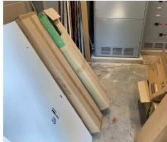
Storage in main electrical room
