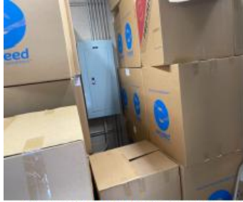
Storage blocking access
