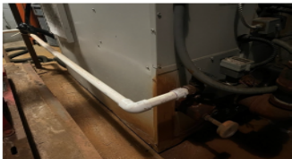
PVC Discharge Piping
