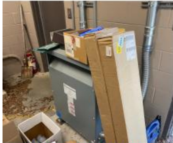
Storage on transformer
