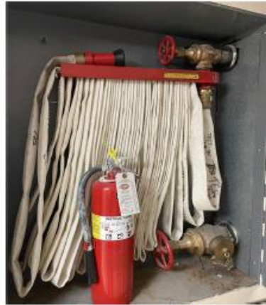
Hose cabinet with extinguisher
