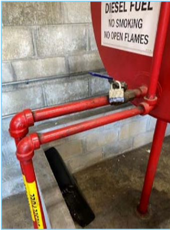
Locked Ball Valve - Diesel Fuel Tank (Diesel Fire Pump)
