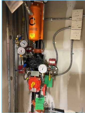
Dry-Pipe Sprinkler Riser
