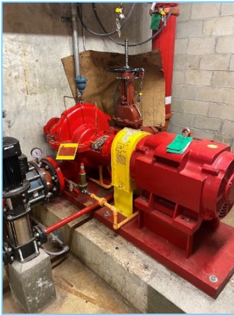
Electric Fire Pump
