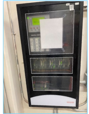
Fire Alarm Panel
