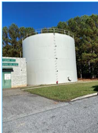
Fire Protection Water Storage Tank (Full)
