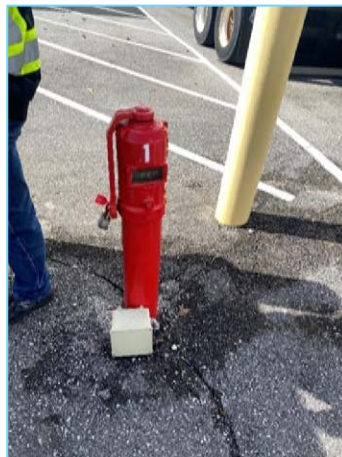
Locked in the Open Position Post Indicator Valve
