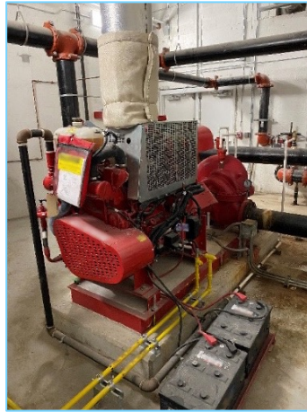
Diesel Fire Pump
