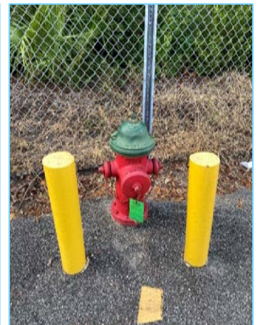
Private Fire Hydrant
