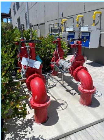
Locked in the Open Position Back Flow Preventers
